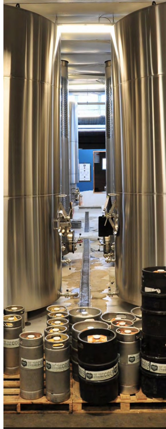
200 BBL Bright Cider Tanks; photo courtesy of Schilling Cider
